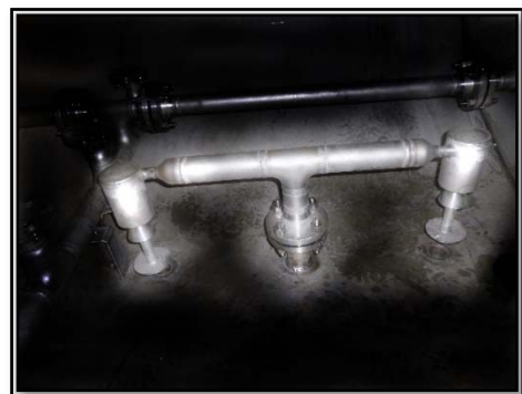
Figure 10: Paired nozzles located above drain nozzles in a degasser vessel.
