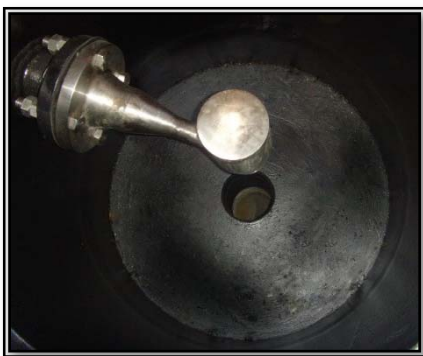
Figure 9: Single nozzle for jetting a solids collection boot under a CPI Plate pack.
